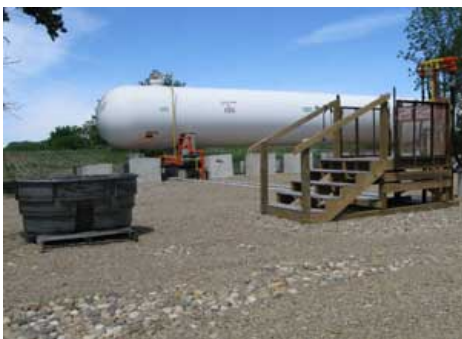
Anhydrous Ammonia installation
